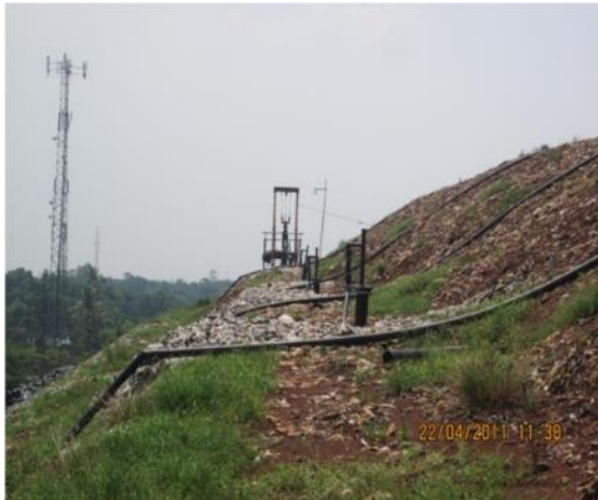
Photo 1: Landfill gas flare (Open Type)
