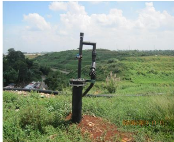
Photo 2: Landfill gas to electricity generation
