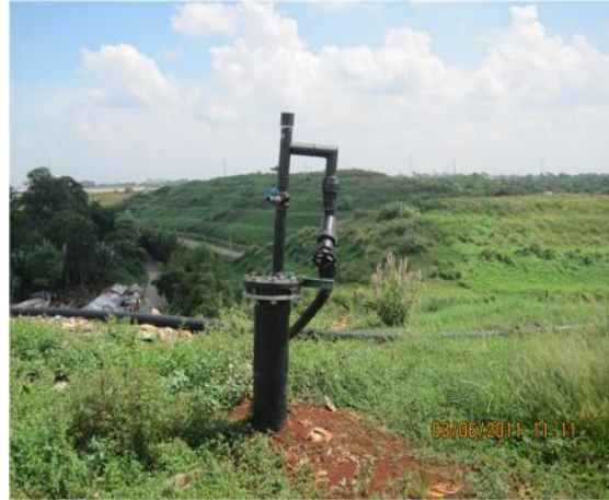
Photo 2: Landfill gas to electricity generation
